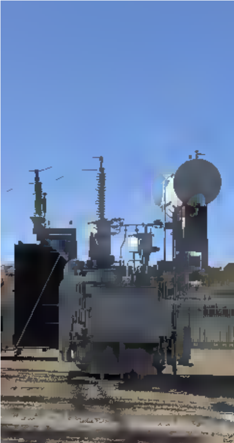
Example of a Transformer
