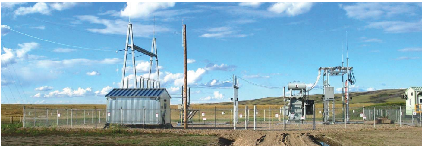
Typical substation in Alberta
